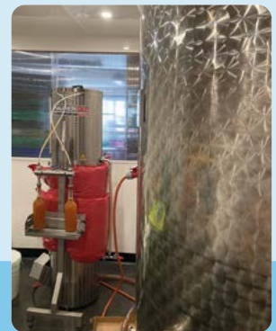
Above: Tamar Grow Local's pasteuriser for their apple juicing facility in Kelly Bray
